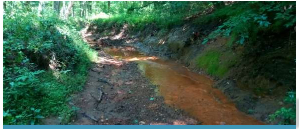
Incised Channel at Broad Creek Park
