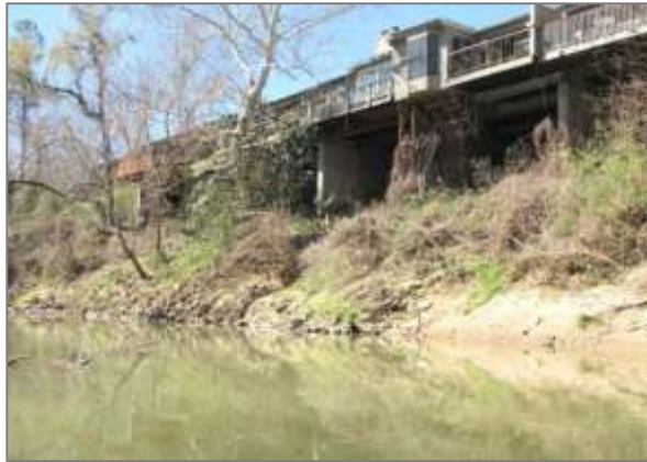
THREAT TO INFRASTRUCTURE
