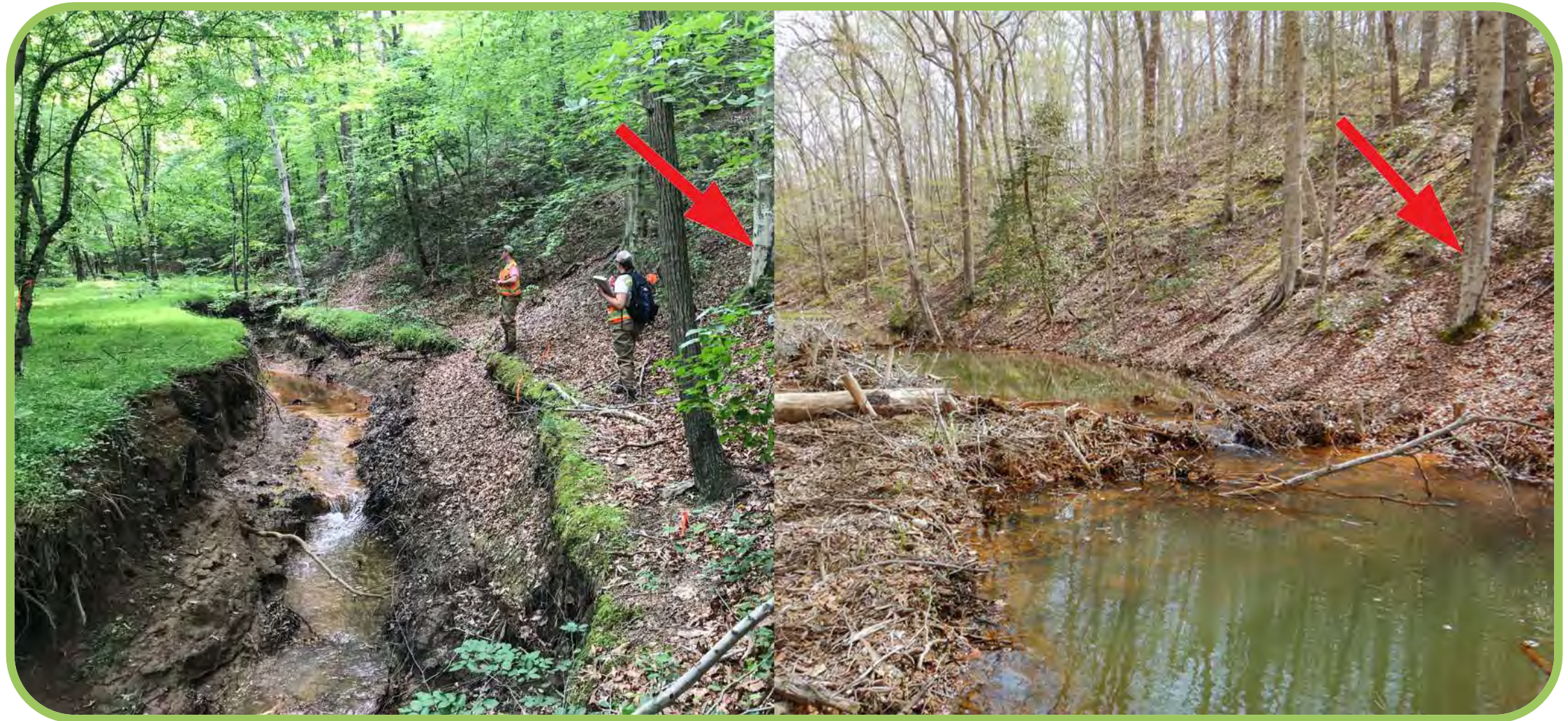
These photos show the increase in stream water surface elevation at the location of a constructed log jam pre- and post-construction.
